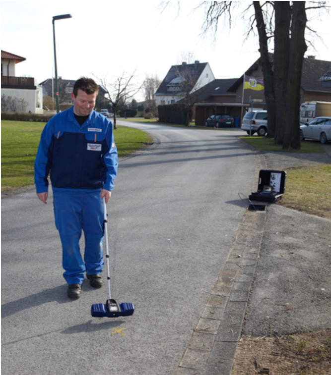
The Wohler VIS 350 precisely locates radio signals transmitted by the camera head through concrete and asphalt to save time and money in repairs.
