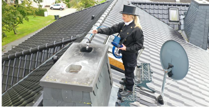
Safe in every position: With the carrying strap system you can inspect easily from the roof.
